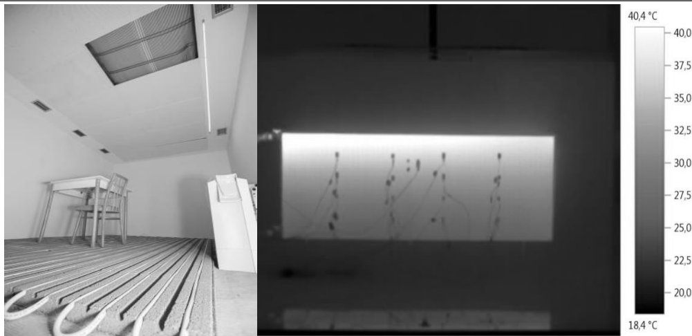
Figure 2: Left: Floor/wall ceiling heating and cooling and fan coil; Right: hot water radiator experiment
