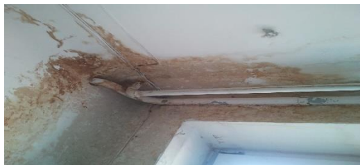
Figure 4 – The microbiological corrosion in industrial building
