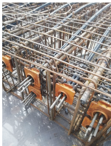
Fig. 2. Anchoring zone of post-tensioned ropes in a monolithic reinforced concrete beam (Construction of the shopping mall in Kyiv)[1]
